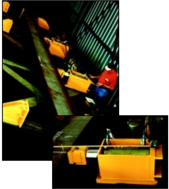
A heavy steel fabricator uses Simplex RDA10012 double acting cylinders to form large sections of I-beam. "The Simplex cylinders and pumps allow us to bend the beams to precise radiuses."
